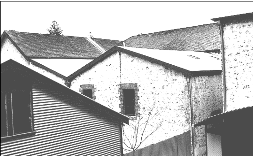
Figure 17: The former Warehouse roof was renovated using materials indicated by the evidence
