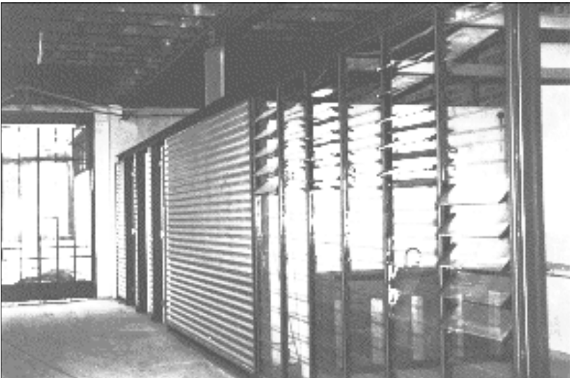
Figure 9: A new wall for the modern facilities constructed on the same plan as a former office wall in the Cartway.
