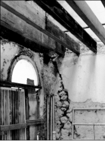
Figure 18: The front facade coming away from the side walls
