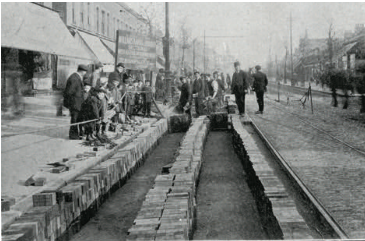
ROMFORD ROAD, EAST HAM, IN COURSE OF CONSTRUCTION WITH SECTIONAL HARD WOOD BLOCKS.
