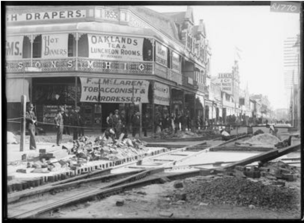
High and Market Street 1905 tram track construction and wooden blocks. From John Dowson's Old Fremantle .
